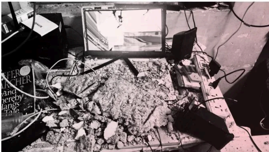
A PICTURE OF THE RESULT OF THE FALLEN CEILING DEBRIS. COURTESY TUSHAR SINGH THAKUR.
